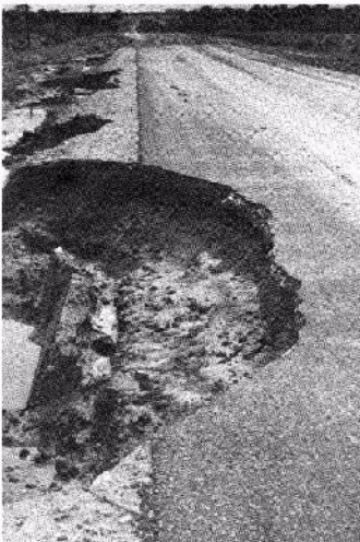
Figure 4-1. Roadway Base Failure
